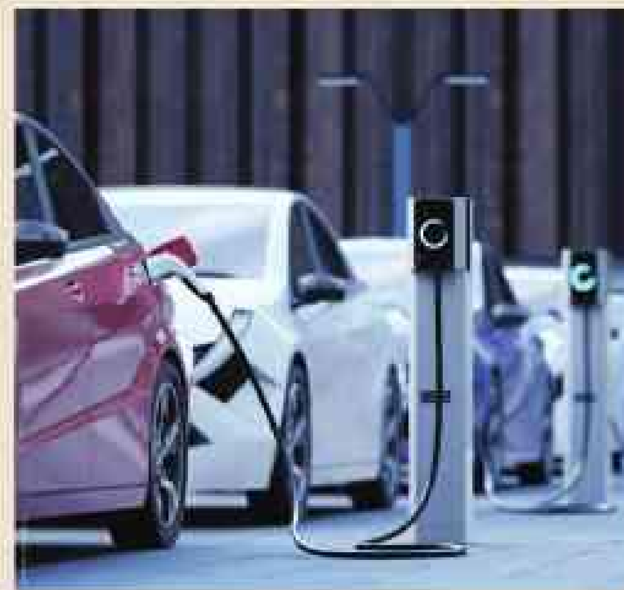
EV Charging Stations
